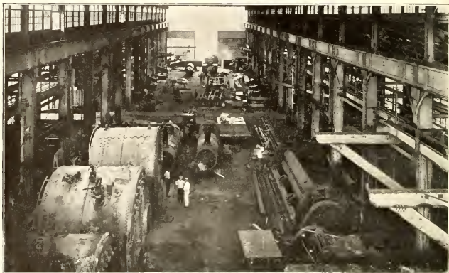
DAMAGED BOILERS FROM GERMAN SHIPS BEING REPAIRED AT BALBOA UNDER DIRECTION OF R. D. GATEWOOD, '06
